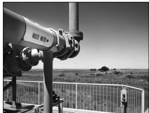
View overlooking Arcata, CA wetland-based wastewater treatment facility
