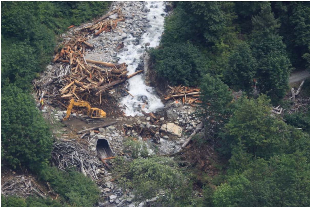
Figure 1. Repair of Boston Creek culvert on Cascade River Road in August 2013. Photo courtesy of the National Park Service.
