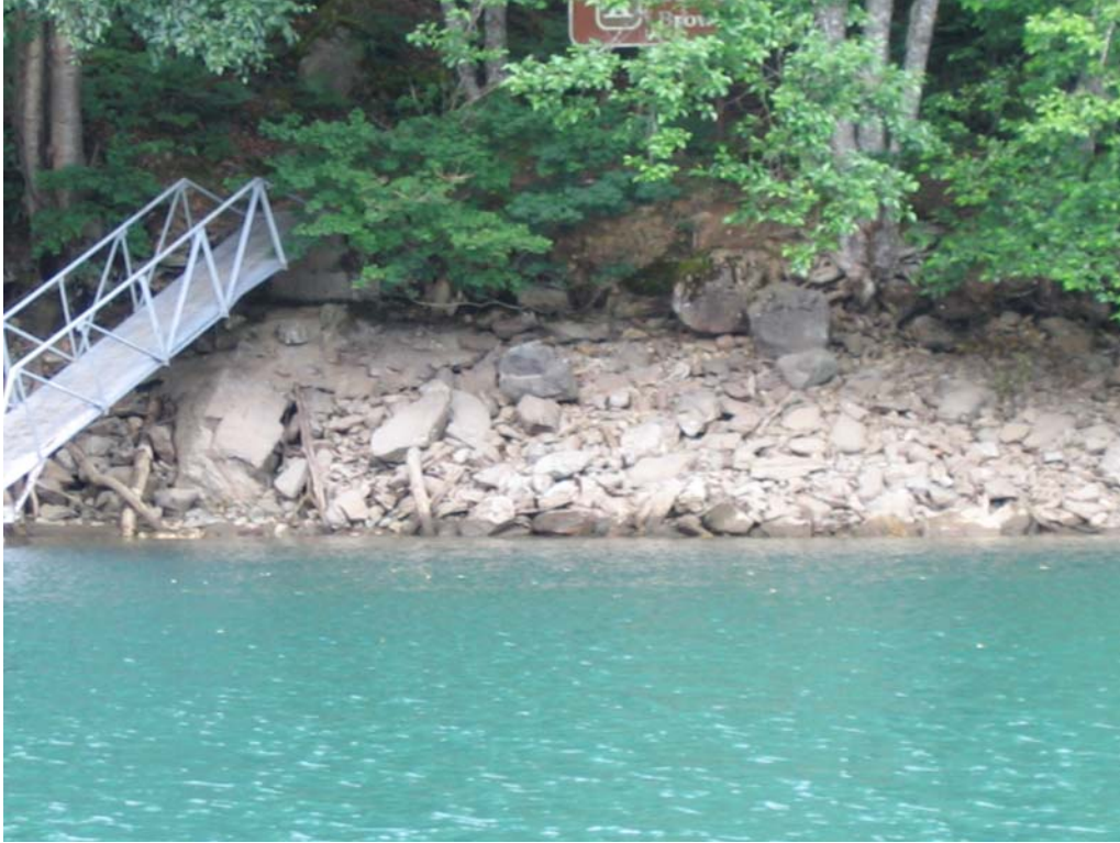
Photo 1: Buster Brown Campground before erosion control measures, June, 2005
