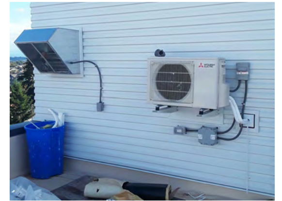
Wall Mounted Pressurization Fan and Elevator Control Room Cooling Unit.
