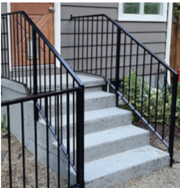
Hot dip galvanized steel guardrail with vertical balusters, painted in black
