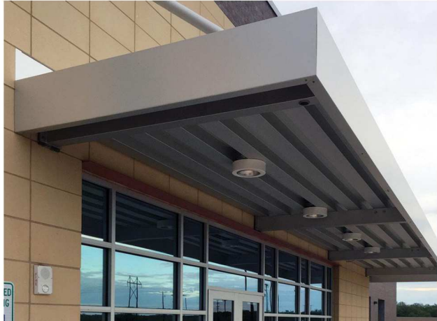
4 OVERHEAD CANOPY LIGHTING
