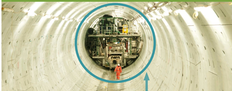
If you look closely, you can see the rings that were placed by this TBM to form the "Lee Tunnel" in London.
