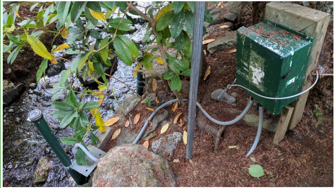
Figure 3. SPU_STA401 Monitoring Station.
