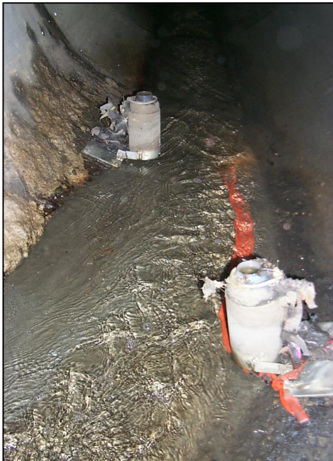
Figure 5: Inline sediment trap.
