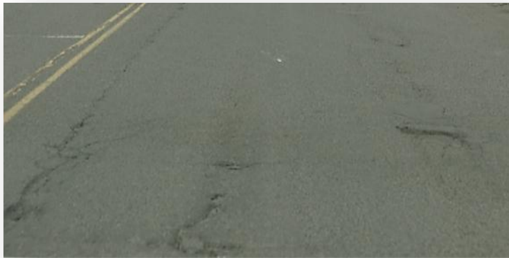
Pavement cracking and spalling. Transpo Group.
