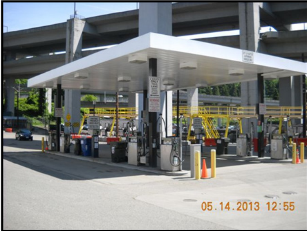
Figure 5. Roof at Fueling Island to Prevent Contact with Rain.
