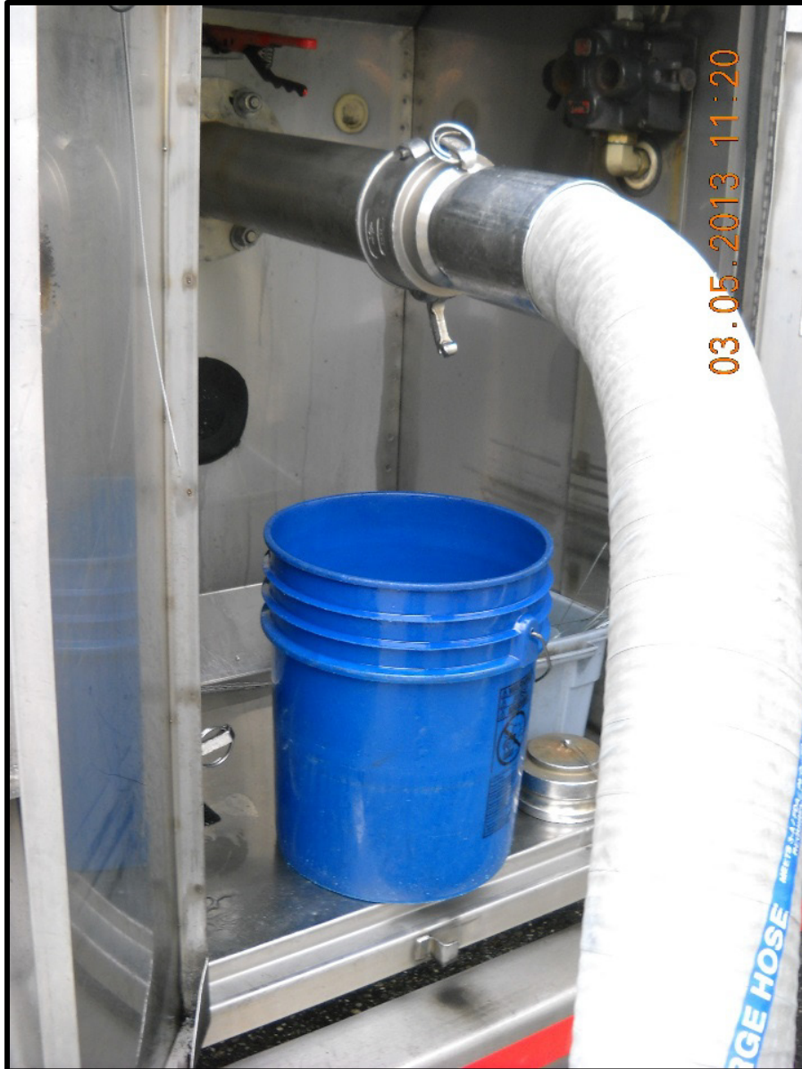
Figure 10. Temporary Containment Device Placed Under a Hose Connection.
