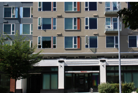
Preservation of the ground floor facade, with a compatible addition above retains a portion of the neighborhood's history.
