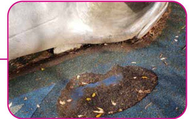
Play surfacing at salmon slide needs repair
