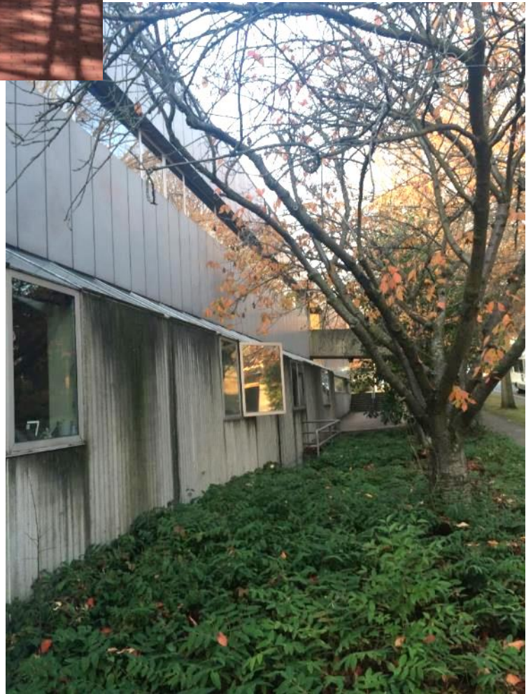
Figure 16. Below, a similar detail view looking north along the first floor east façade, south of the entry ramp.
