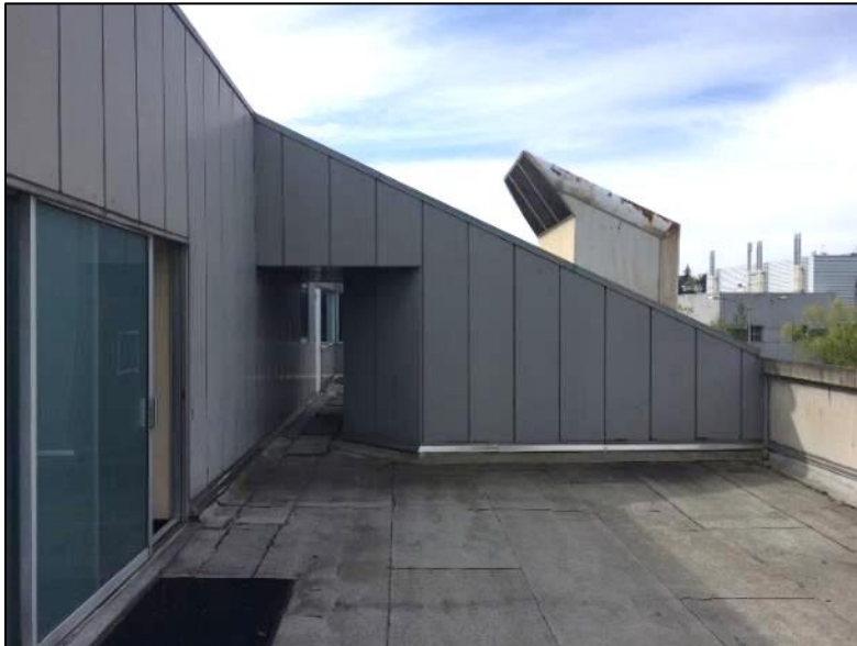
Figure 26. Below, equipment on the 2 nd floor west roof setback.
