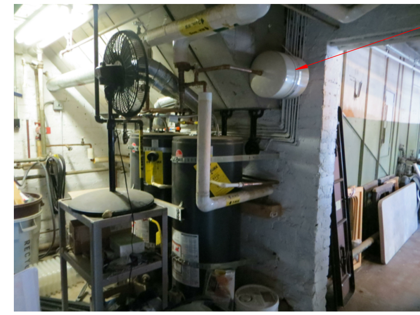
(E) TANK CONFLICTS WITH PROPOSED HALL CLEARANCE
