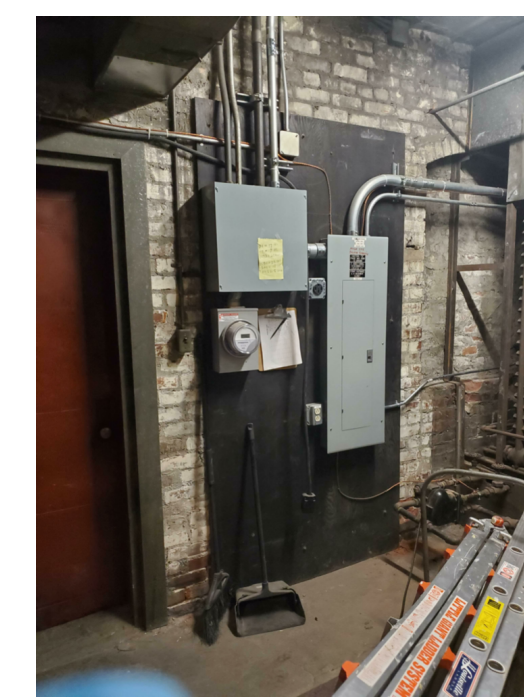
EXISTING SERVICE PANEL
