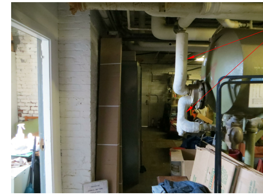
(E) TANK AND PIPES CONFLICT WITH PROPOSED HALL CLEARANCE
