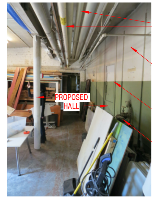
(E) PIPES AT PROPOSED HALL LOCATION (E) DUCT COVER (E) DUCT ACCESS (E) EQUIPMENT AT PROPOSED HALL LOCATION
