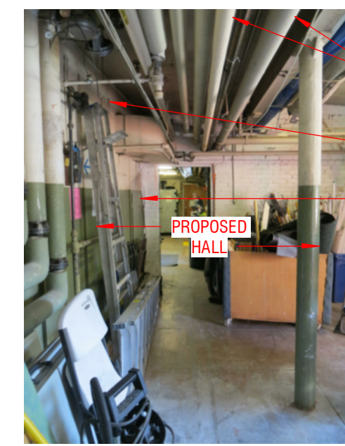
(E) PIPES AT PROPOSED HALL LOCATION (E) DUCT COVER (E) DUCT ACCESS
