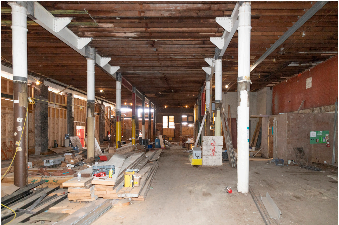
PHOTO 15. After: first floor, 2022, looking through the space with the mezzanine removed and intumescent paint applied to steel.
