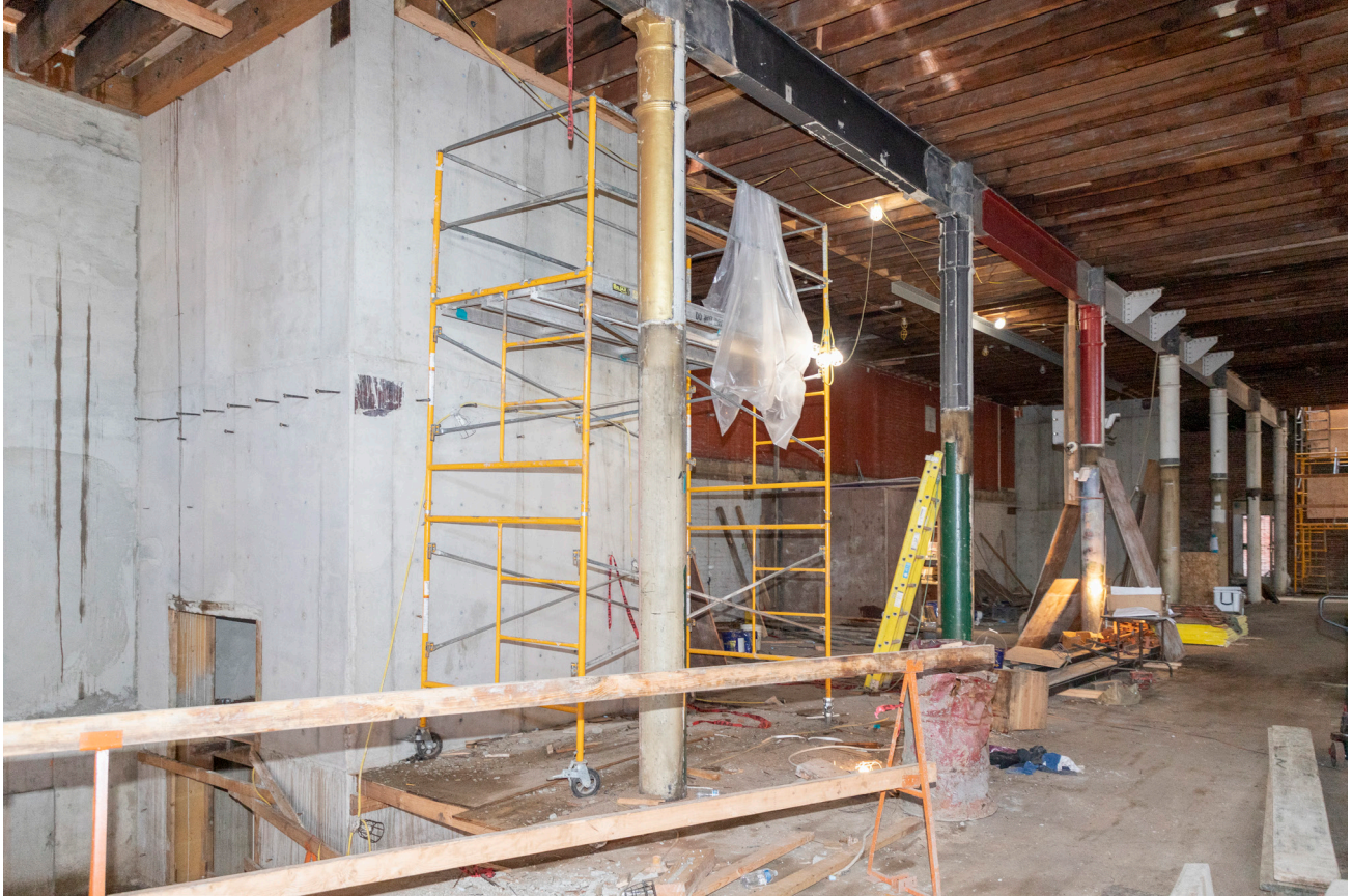
PHOTO 12. After: first floor, 2022, elevator core and completed concrete work for Shear Walls 3-6.
