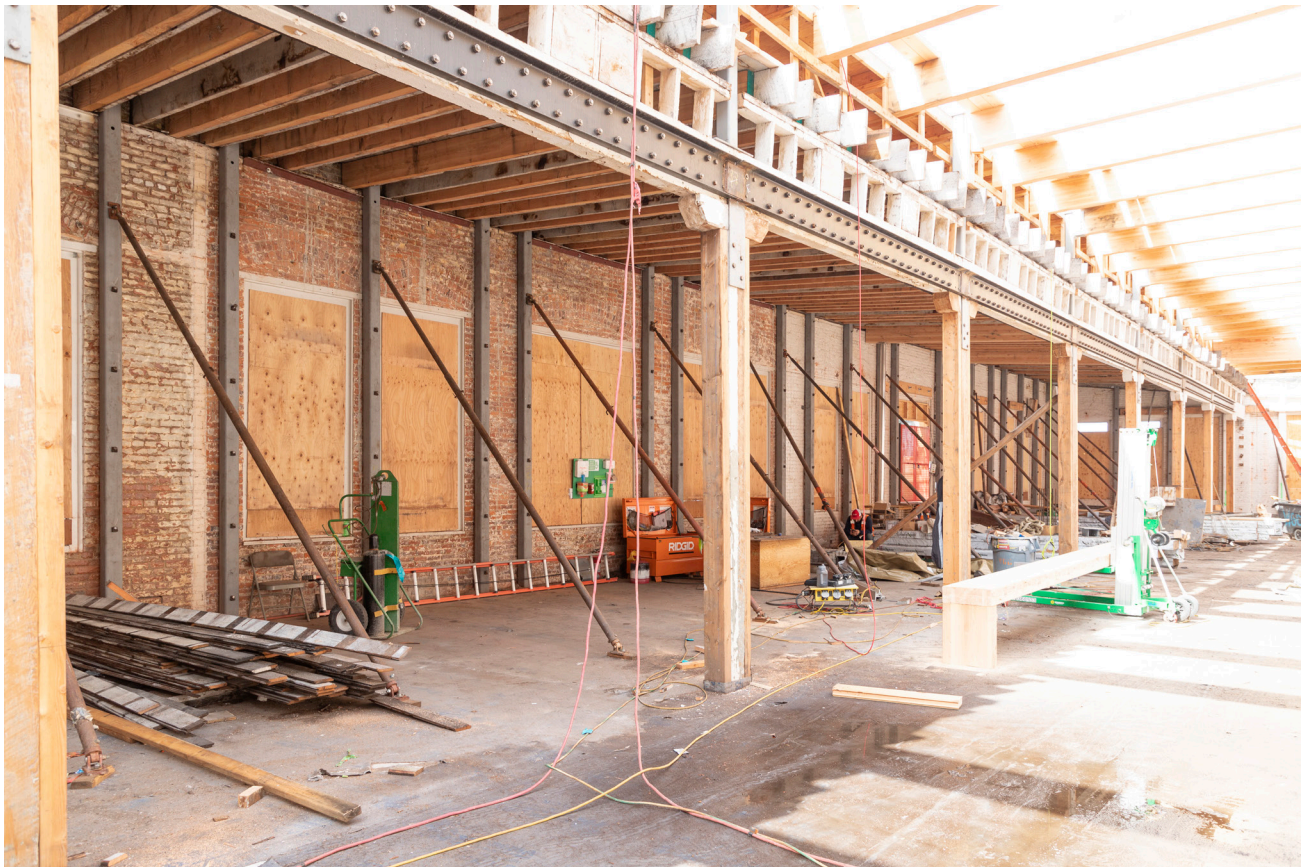
PHOTO 27. After: 2022 third floor, showing seismic retrofit steel at columns and strong backing at brick completed.
