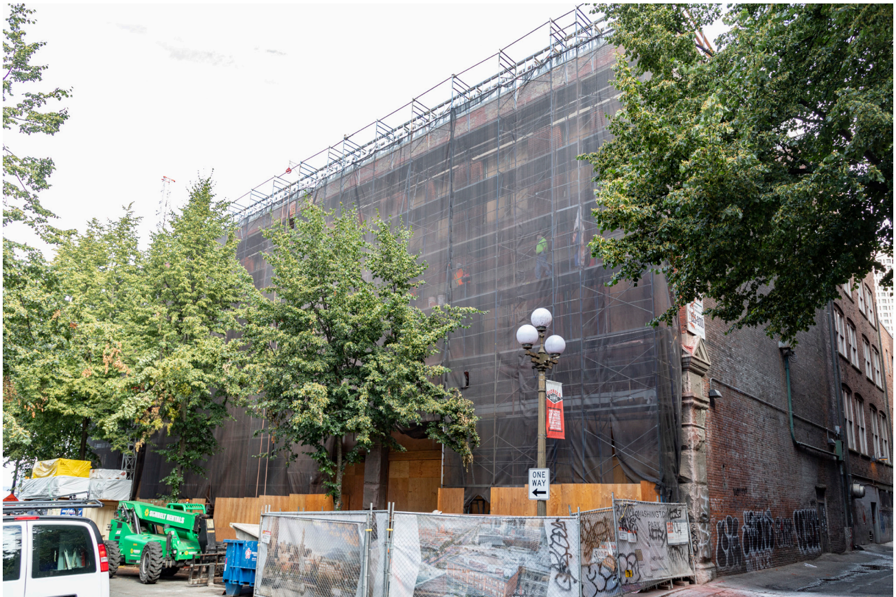
PHOTO 2. After: 2022 site, showing construction fencing, temporary protection at the storefronts, and repointing work under way.
