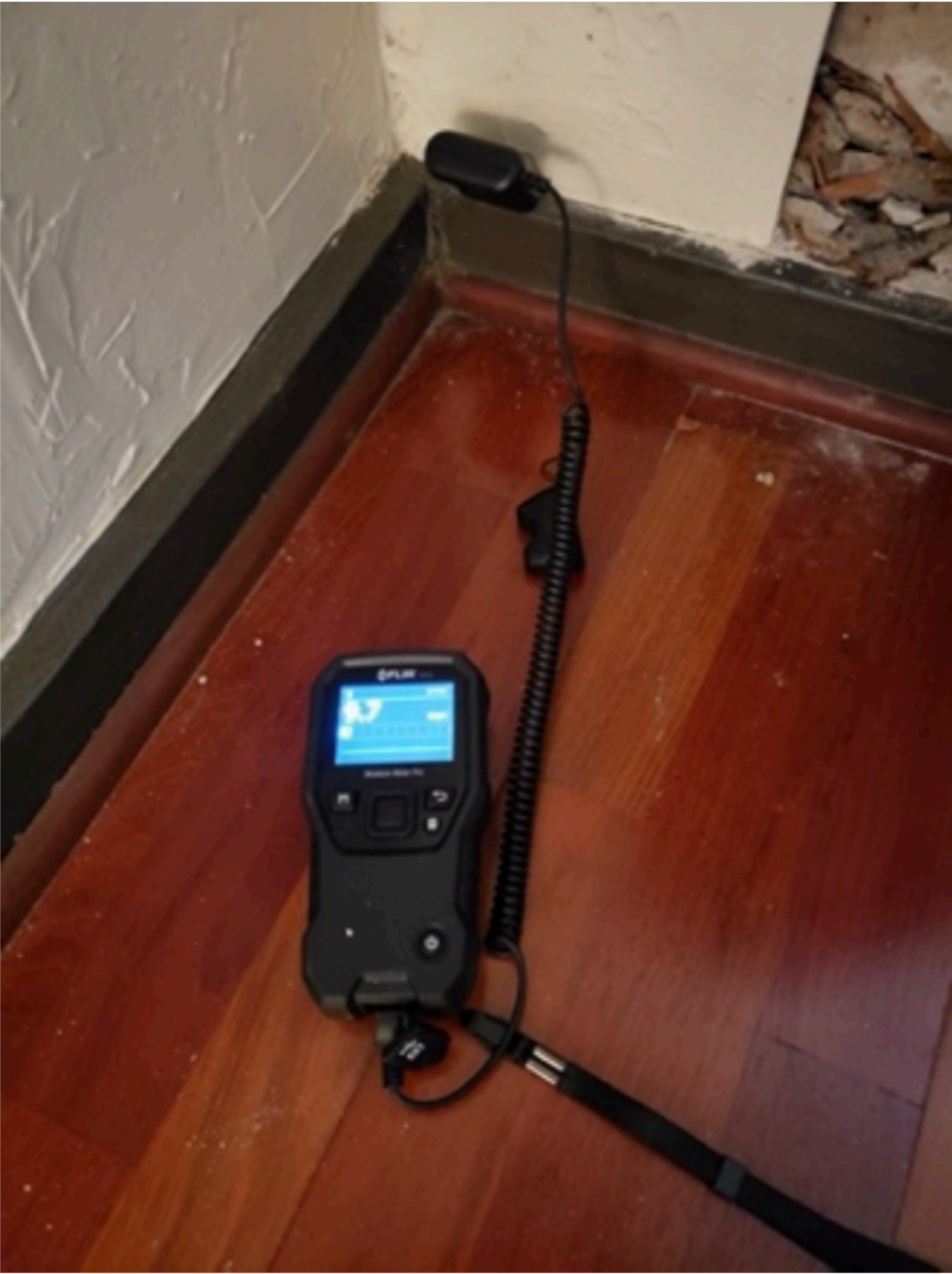
Elevated moisture readings at test location
