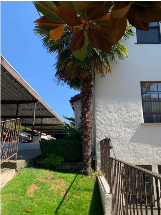
Base of tree 8" from building
