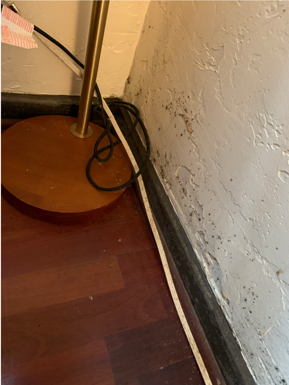
Mold growth at Northwest corner of Unit 107
