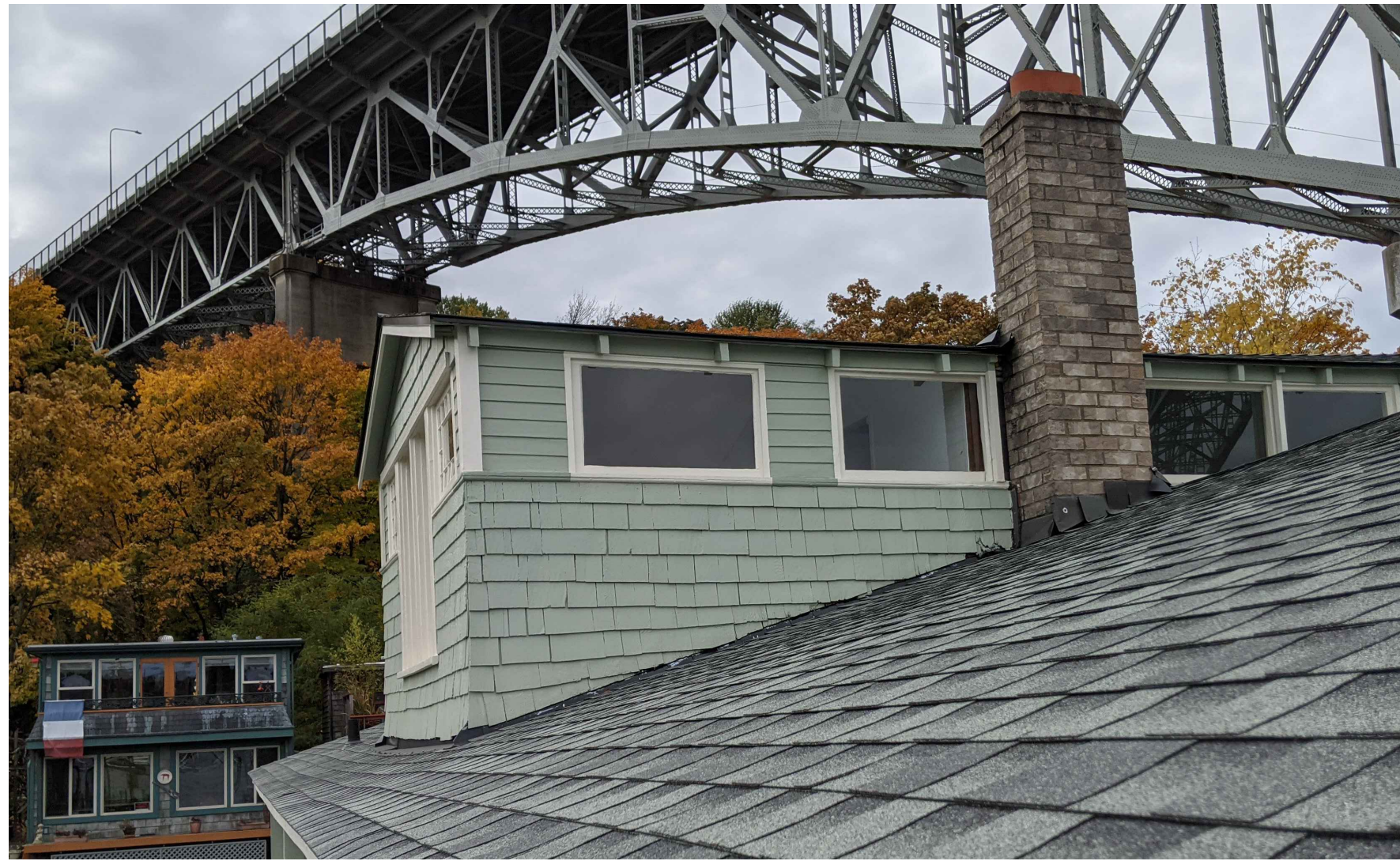
NORTH - 1 (ALL PHOTOS BY JAS SITE VISIT 10/20/2021 - UNLESS NOTED OTHERWISE)
