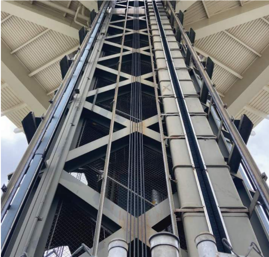
Existing hoistway equipment
