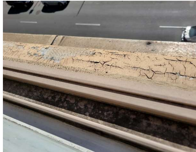
Failed sill repair
