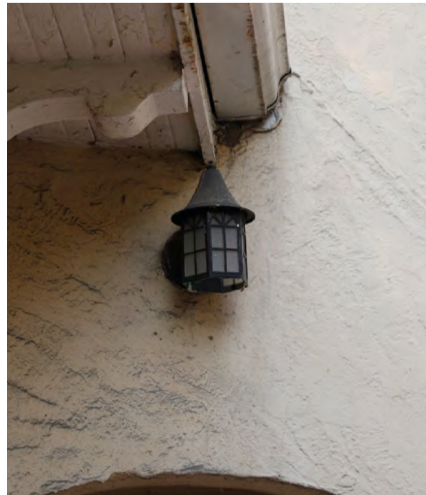
Figure 82. Wall bracket lantern detail.
