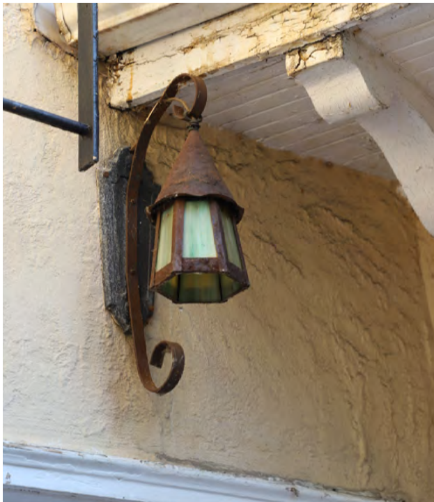
Figure 80. Wall bracket lantern detail.
