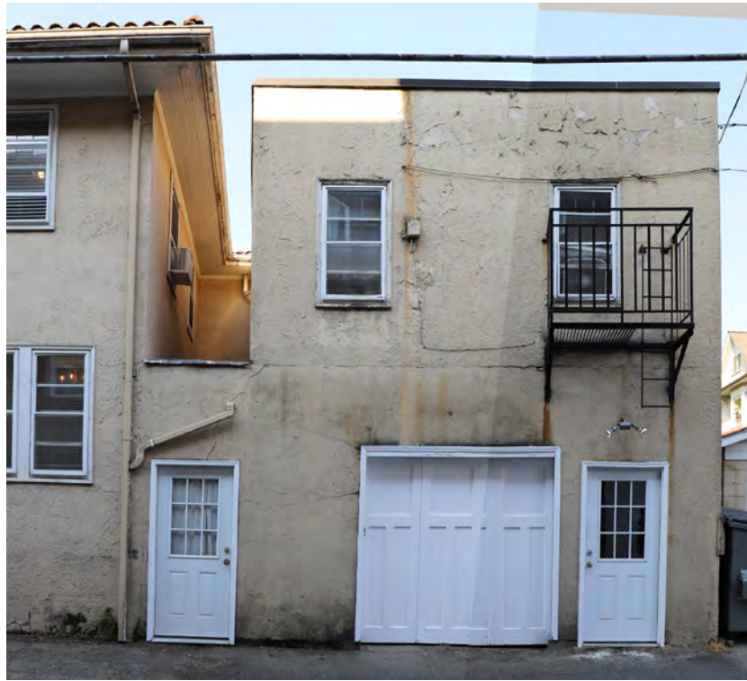
Figure 22. Exterior, northeast corner, east facade. Composite image showing metal balcony at apartment, garage door, and light well.
