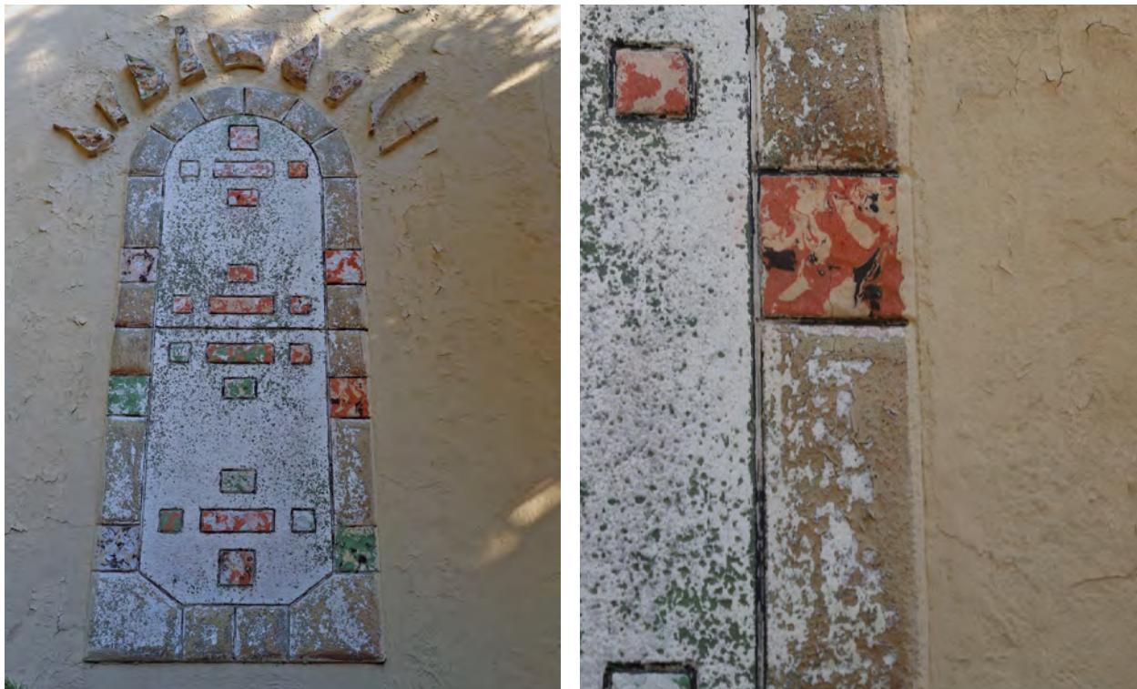
Figure 24. End wall applied decorative element details. Overall view (above left) and detail (above right) and detail (below left).
