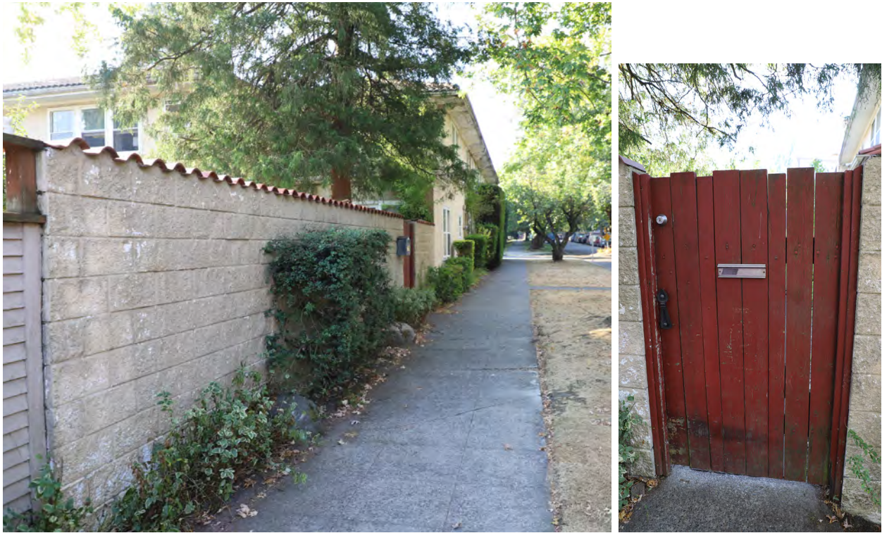
Figure 14. Backyard, west wall. Concrete block wall looking south (above left) and gate (above right).
