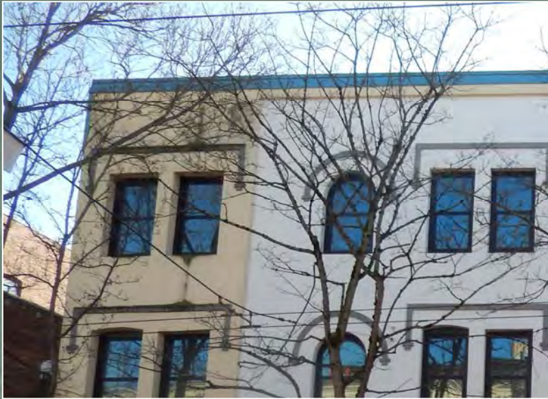
Northeast Corner – Missing Parapet and Frieze
