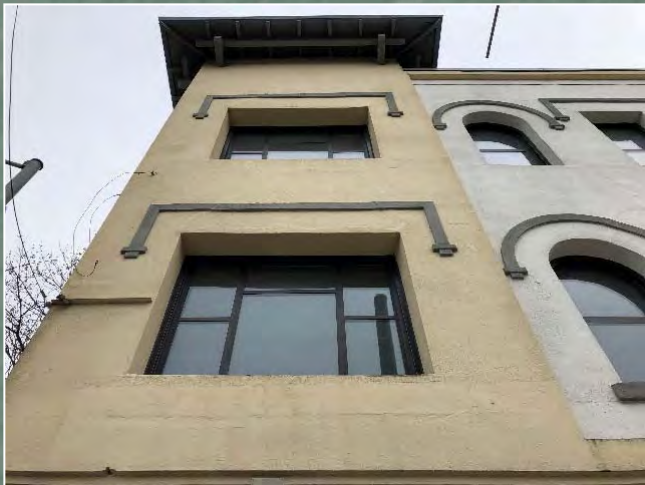
Northwest Tower Detail – Windowsills and Quatrefoil Missing
