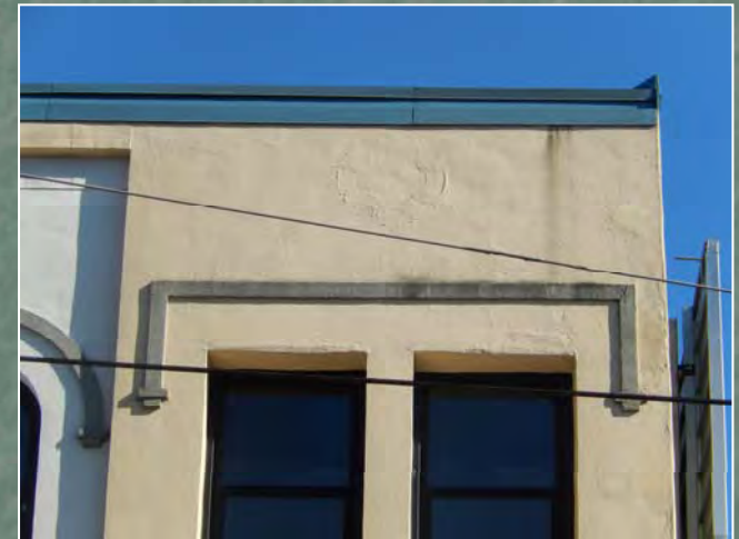
South Corner – Cornice Frieze, Scalloped Parapet and Coping, and Quatrefoil Missing
