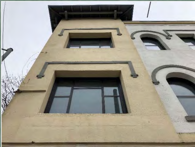
Northwest Tower Detail – Windowsills and Quatrefoil Missing
