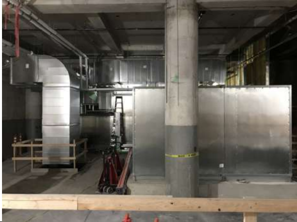
SB Mechanical Room
