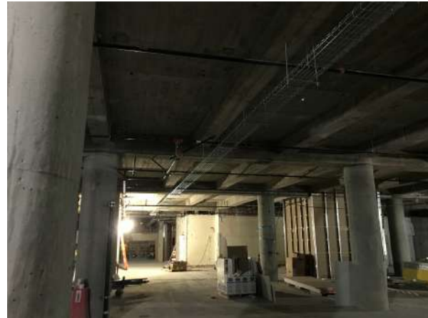
Metro Cable Tray/Fire Suppression
