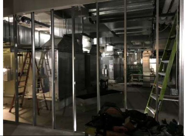
SB Mechanical Room
