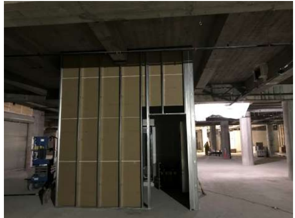
Metro Electrical Room Typ.
