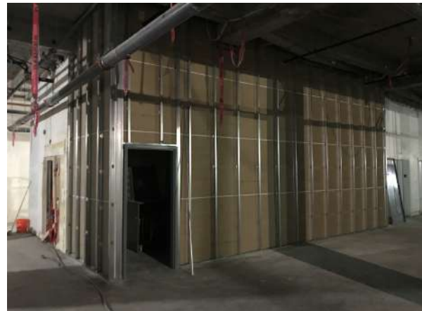
L2 Electrical Room
