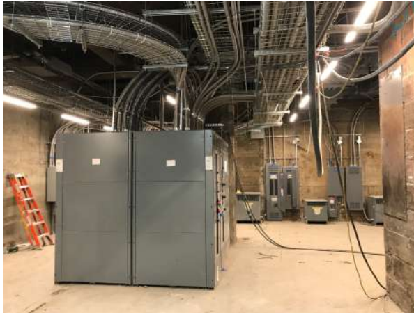
SB Electrical Room
