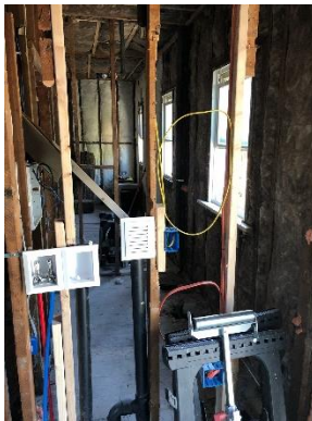
Unit 2 Laundry Plumbing and Coax panel
