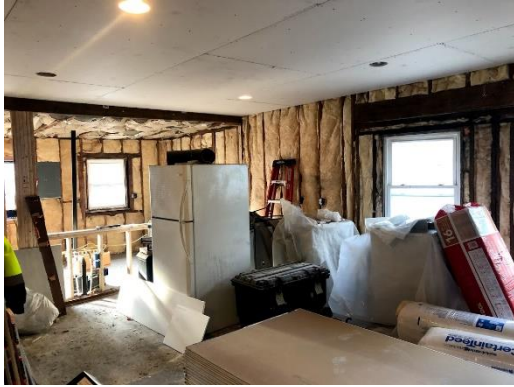
Insulation, Ceilings, and Electric Panel
