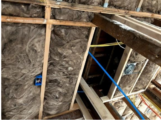
Upstairs Kitchen supply lines Running from Unit 2 Downstairs Drop Ceiling Framing and insulation
