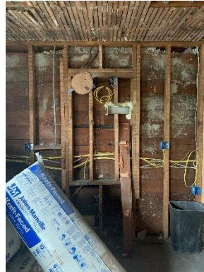
Unit 1 Kitchen Electrical
