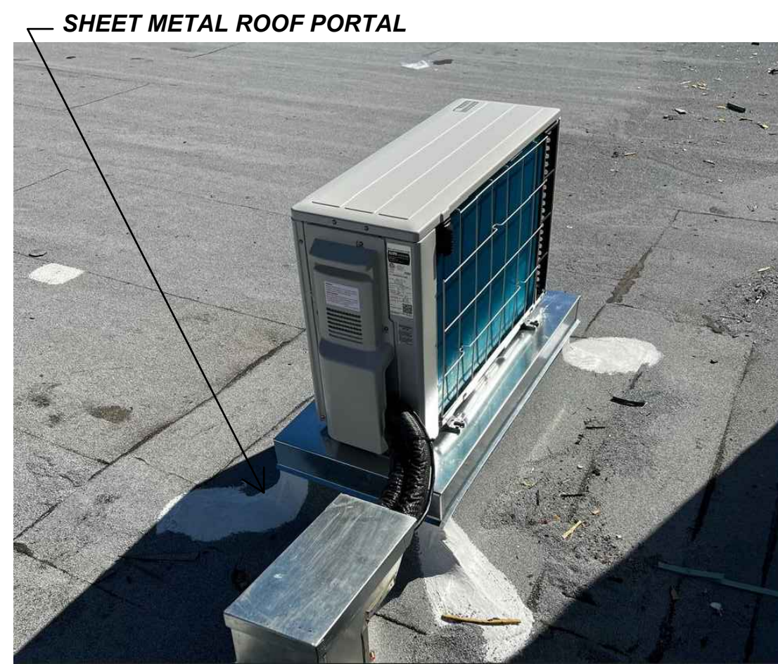
ROOFTOP HEAT PUMP OUTDOOR UNIT (MINI SPLIT HP-3&4)
