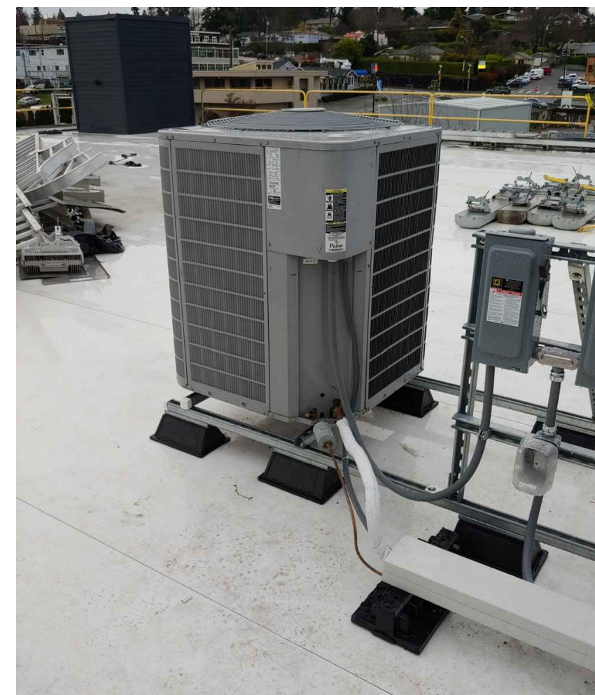
ROOFTOP HEAT PUMP OUTDOOR UNIT (HP-1A, 1B, & 2)
