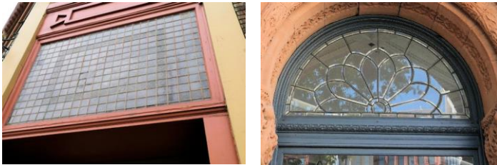
Figure xxx/ Pioneer Square buildings often feature unusual decorative windows that should be retained.
