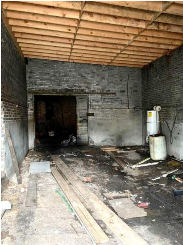
Left, an interior view of one of the service bays in the Garage in 2021 (photograph by Anton Dekom, Neiman Taber Architects).
