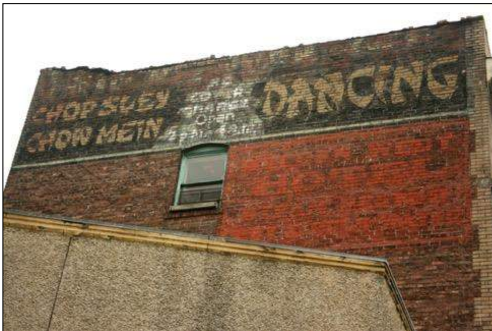
Below, a 2008 photo of painted signage on the upper north façade of the Republic Hotel, showing and the condition of the masonry and parapet. The stucco clad walls in the foreground are part of the subject garage.
