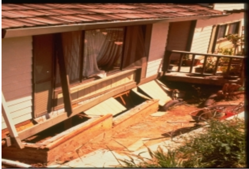
Figure 3. Home moved off the foundation wall (photo from Applied Technology Council)
