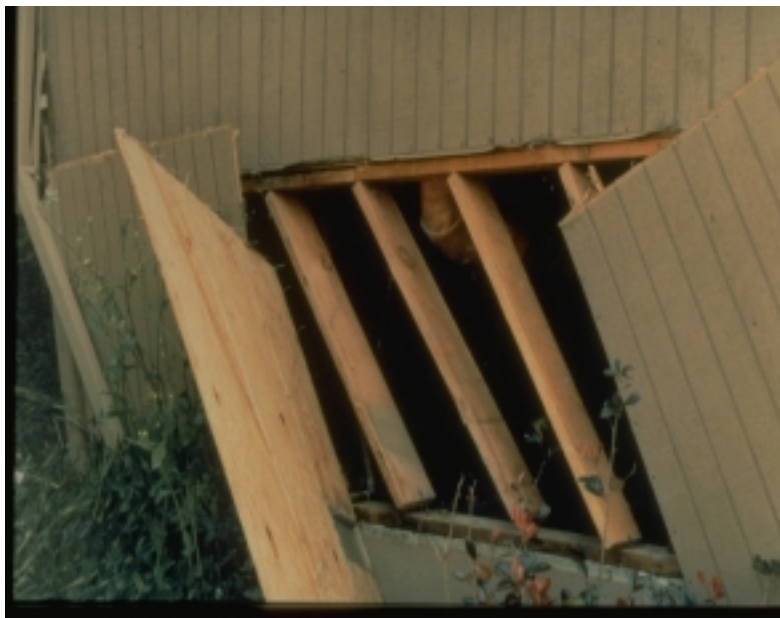
Figure 4. Collapse of the short wall between the first floor and the foundation (photo from Applied Technology Council)
