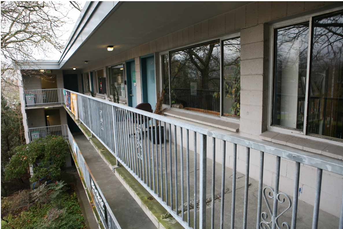
Photograph 38: View along 3rd floor balcony, looking west, Blue Spruce Building. Courtesy Artifacts Consulting, Inc.
