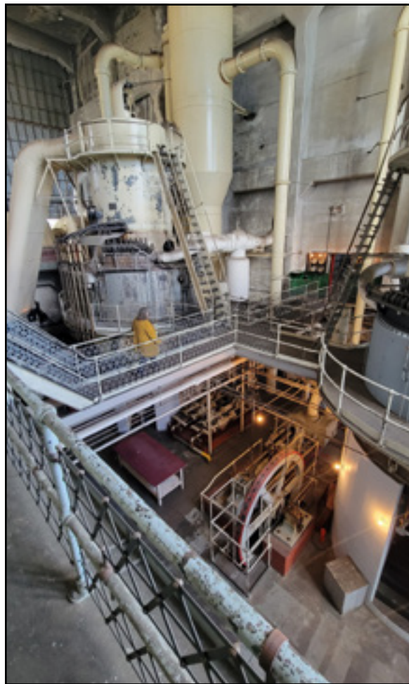
Georgetown Steam Plant [photos: Kate Clark]
