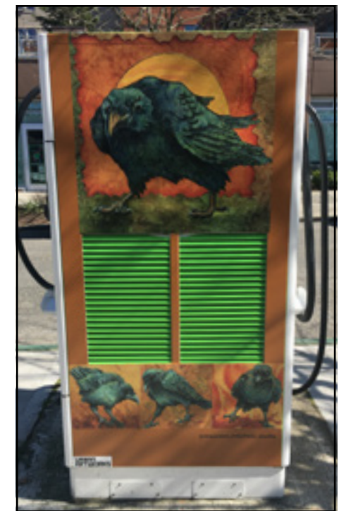
Maureen Mitchell, Seattle City Light Beacon Hill electric vehicle service cabinets.
