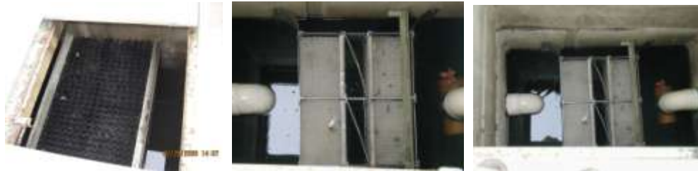
Oil/Water Separator (coalescing plate)
