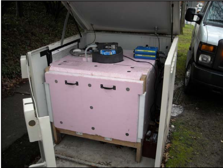
Figure 2.2.2.b. Photograph of C1 Equipment Cabinet
