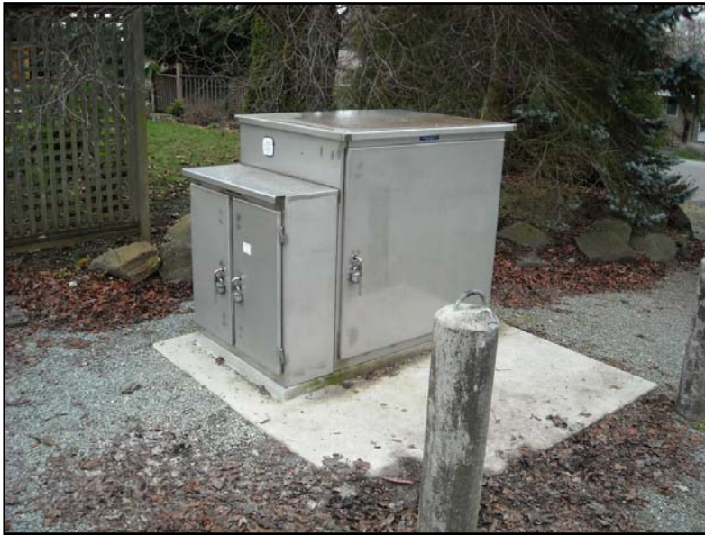
Figure 2.2.2.1c. Photograph of R1 Equipment Cabinet
