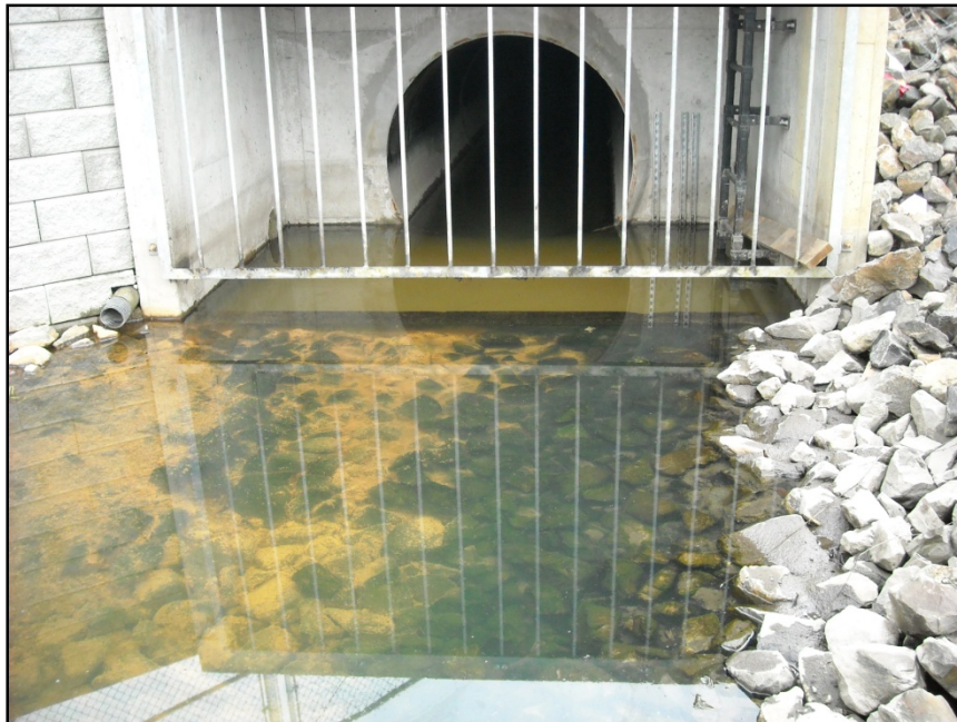
Figure 2.2.2.3c. Photograph of I1 Diversion Structure and Outfall
