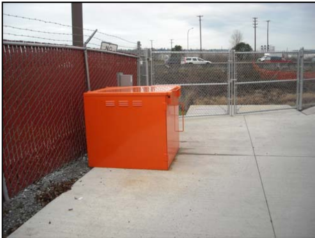
Figure 2.2.2.3d. Photograph of I1 Equipment Cabinet
