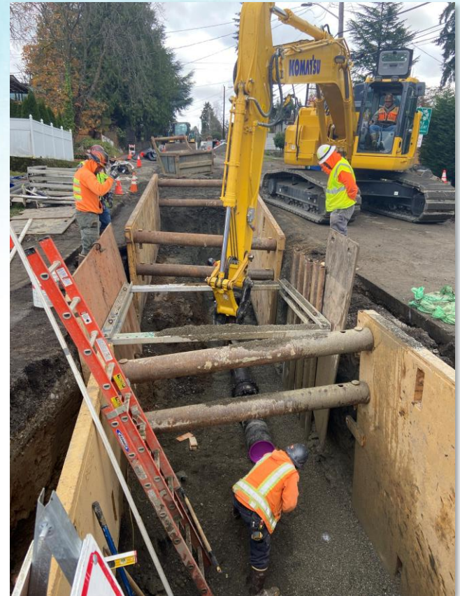
A Drainage Rehab project located on NE 92nd St. This project replaced a failing drainage mainline
