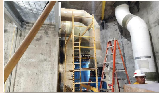
Photo (left): Inside the Fremont Shaft, showing piping and ducting under construction.
