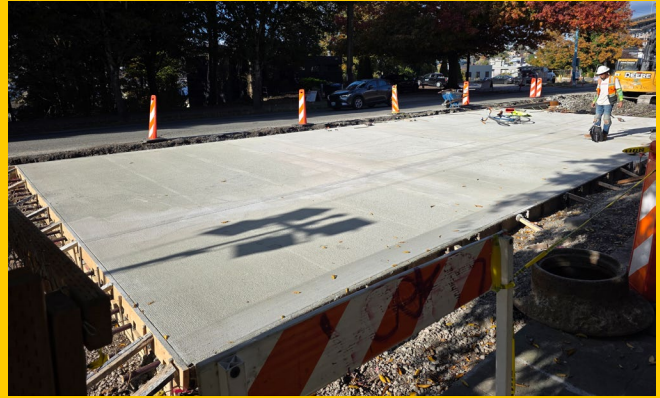
J Line: new full-depth concrete panels that provide a long-lasting street surface to withstand heavy use from RapidRide buses
