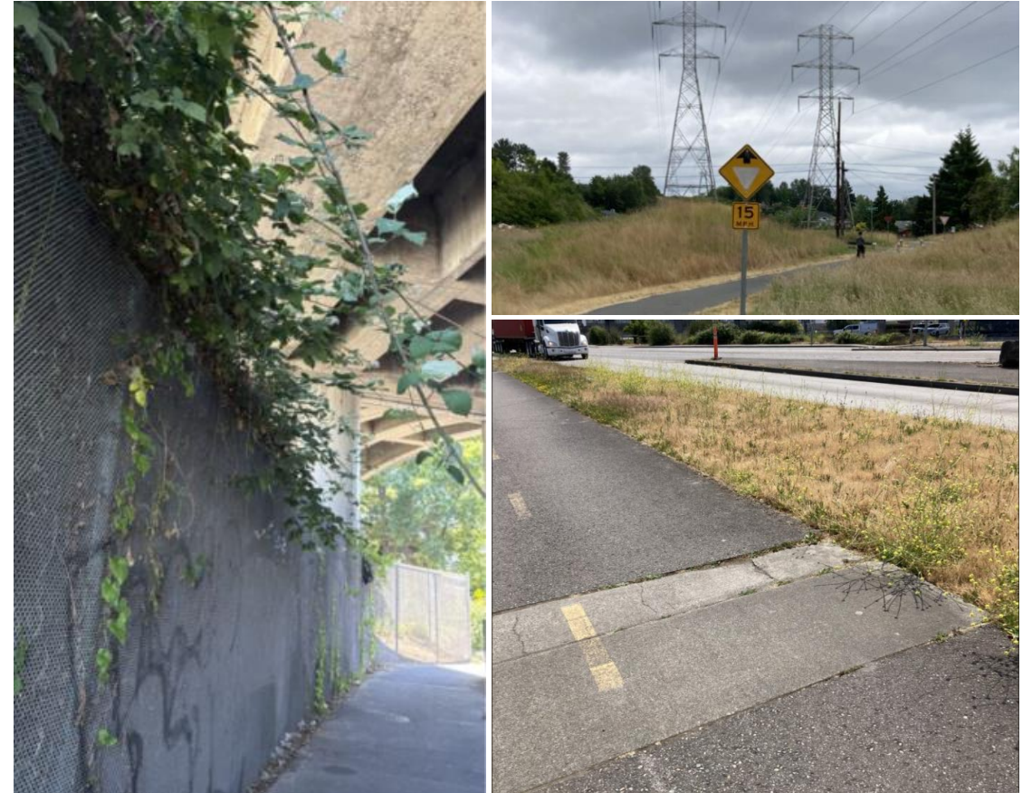
Faded signs, intruding blackberries, and separation of pavement are examples of minor trail issues
