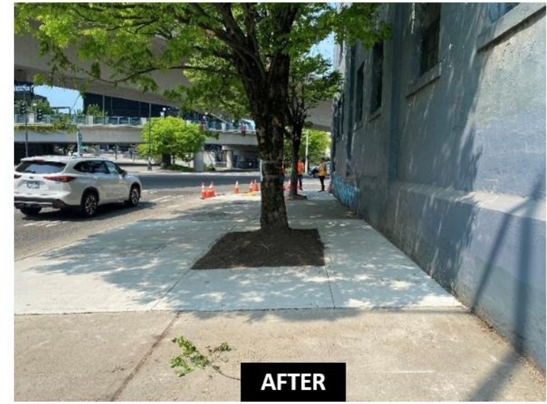
Before (left) and after (right) of sidewalk repair on 4th Ave S & S Royal Brougham Way.
