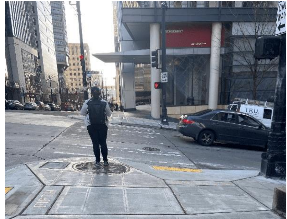
Bottom: New ADA curb ramps at 5th Ave and Madison St at part of Madison RapidRide G Line project.
