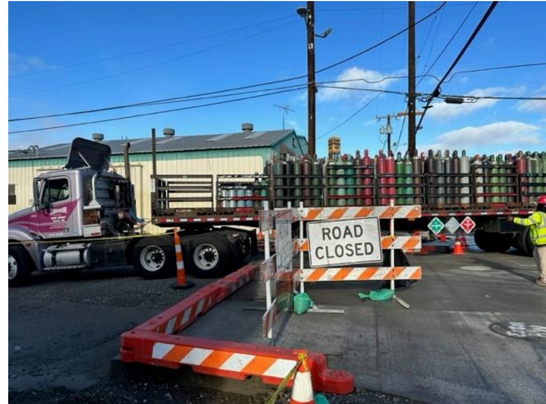
Traffic control as part of this project ensuring truck access to local businesses during construction
