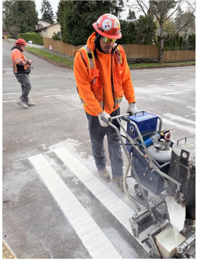
SDOT crews remarking crosswalks on SW Myrtle St and 16th Ave SW.
