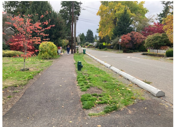
New walkway on Corliss Ave N between N 117th and N 120th streets near James Baldwin Elementary School.
