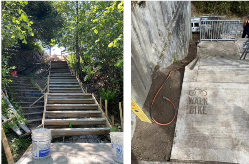
California Pl SW stairway under construction (left) and Princeton Ave NE stairway bike runnel (right).
