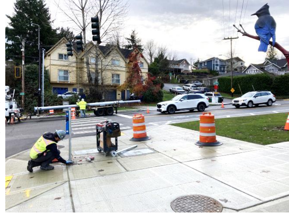
Program 1 - Work in progress at the SW Holden St and Highland Park Way SW intersection, including traffic signal mast arms, new sidewalks, and ADA-accessible curb ramps. Also shown is a new sculpture, Where's the Party: Elevating Nature and Resilience, a fiberglass representation of a Steller's Jay .
