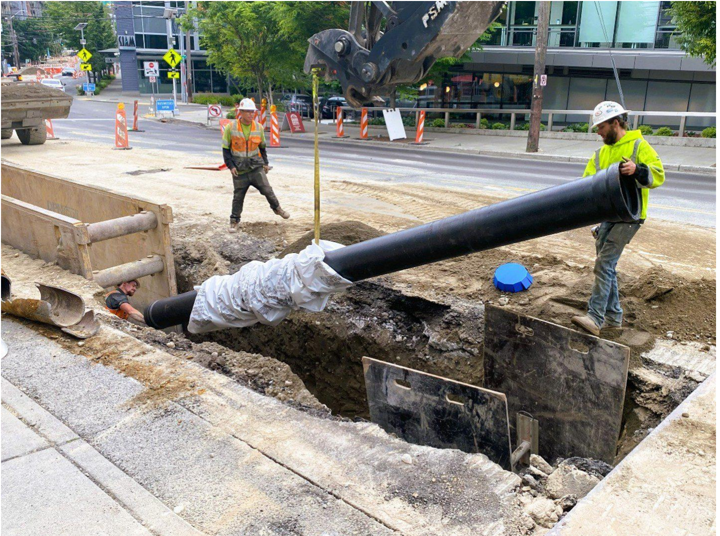
Crews install a new water main pipe on Eastlake Ave E as part of the RapidRide J Line project.
