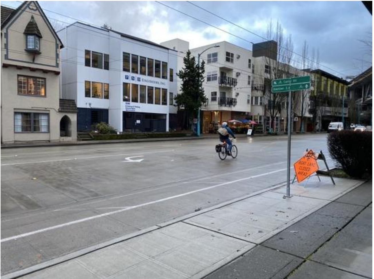
Bicyclist rides across new concrete on Eastlake Ave E as part of the RapidRide J Line project.
