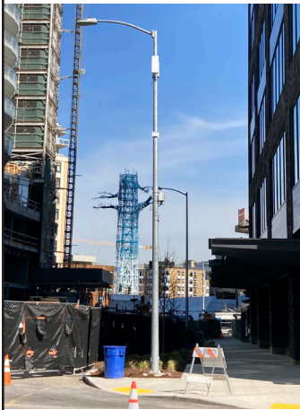
Image 4: Metal pole with side-mount panel antennas and disconnect
