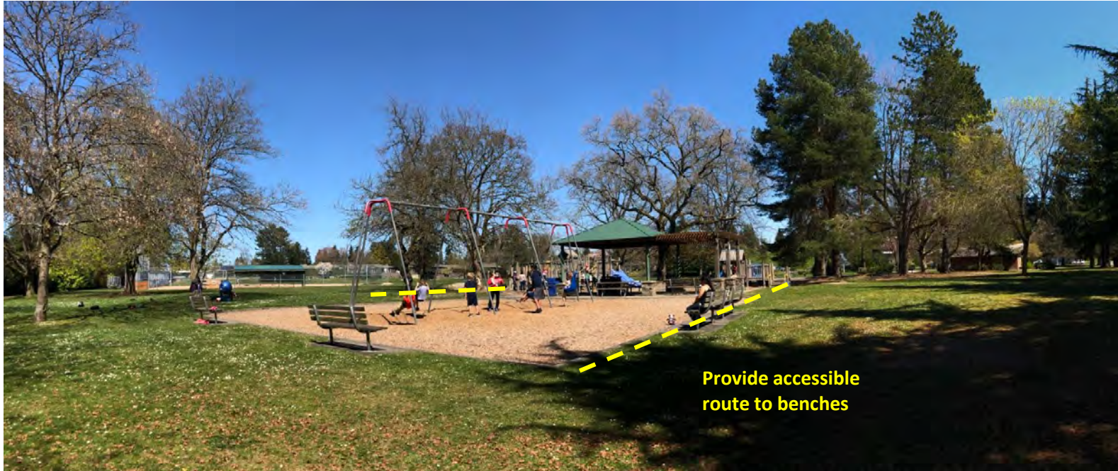
Existing tall swing is aging & exceeds maintenance height. Toddler bucket swing exceed maximum 8' high. Lack of accessible route to existing benches.
