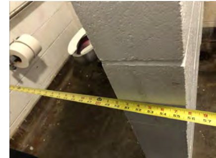
Accessible compartment is too small in restroom.
