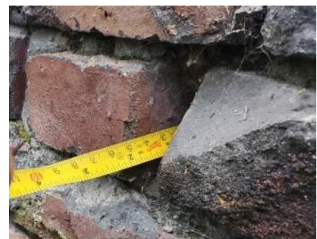
Mortar Bed Erosion at Masonry
