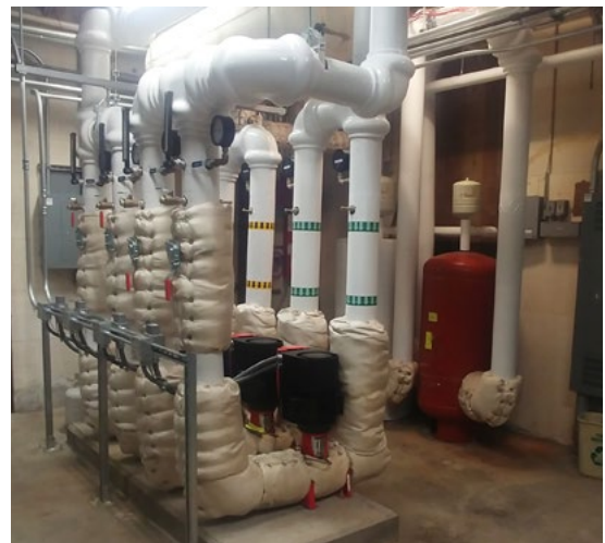
Hydronic pumps for supply and return chilled and heating water. Credit: WA DES
