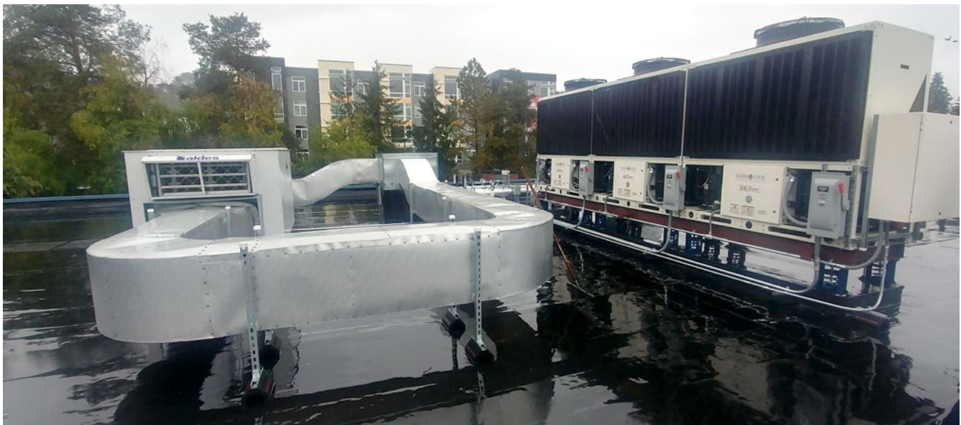
The new air source heat pump with DOAS. Credit: WA DES
