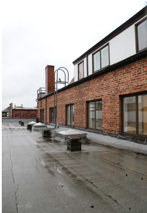
Figure 40. Roof over the southwest portion looking west along the back side of the north ell.
