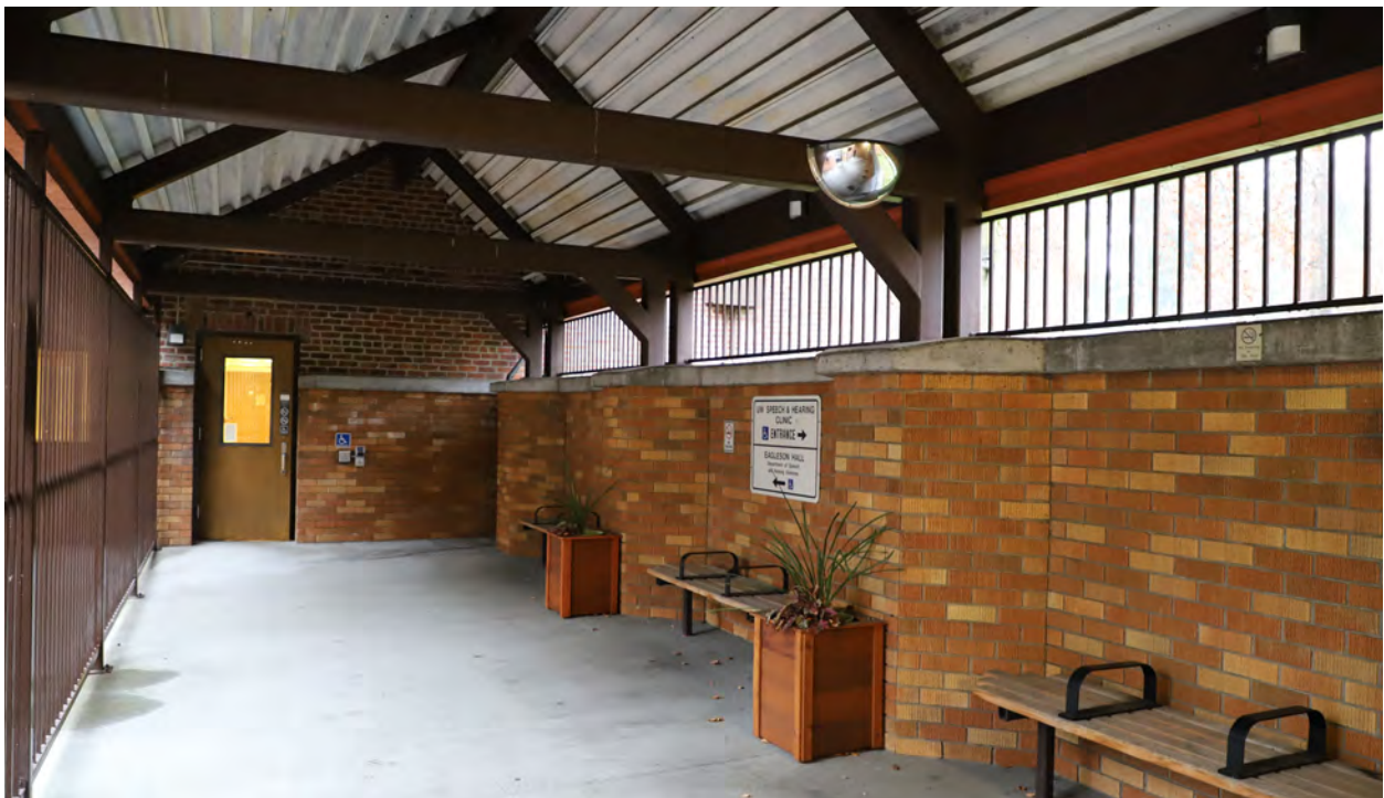
Figure 28. Covered breezeway connection on the south facade, looking north towards the building.
