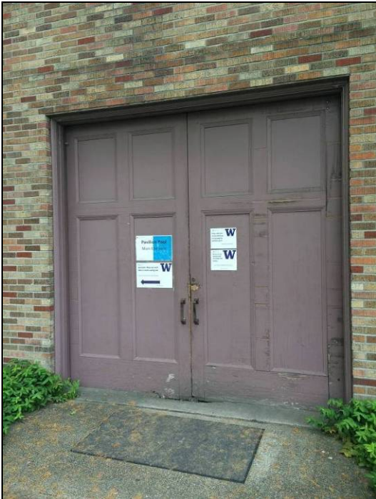
Figure 18. Below, detail view of a service entry at grade level, east facade.
